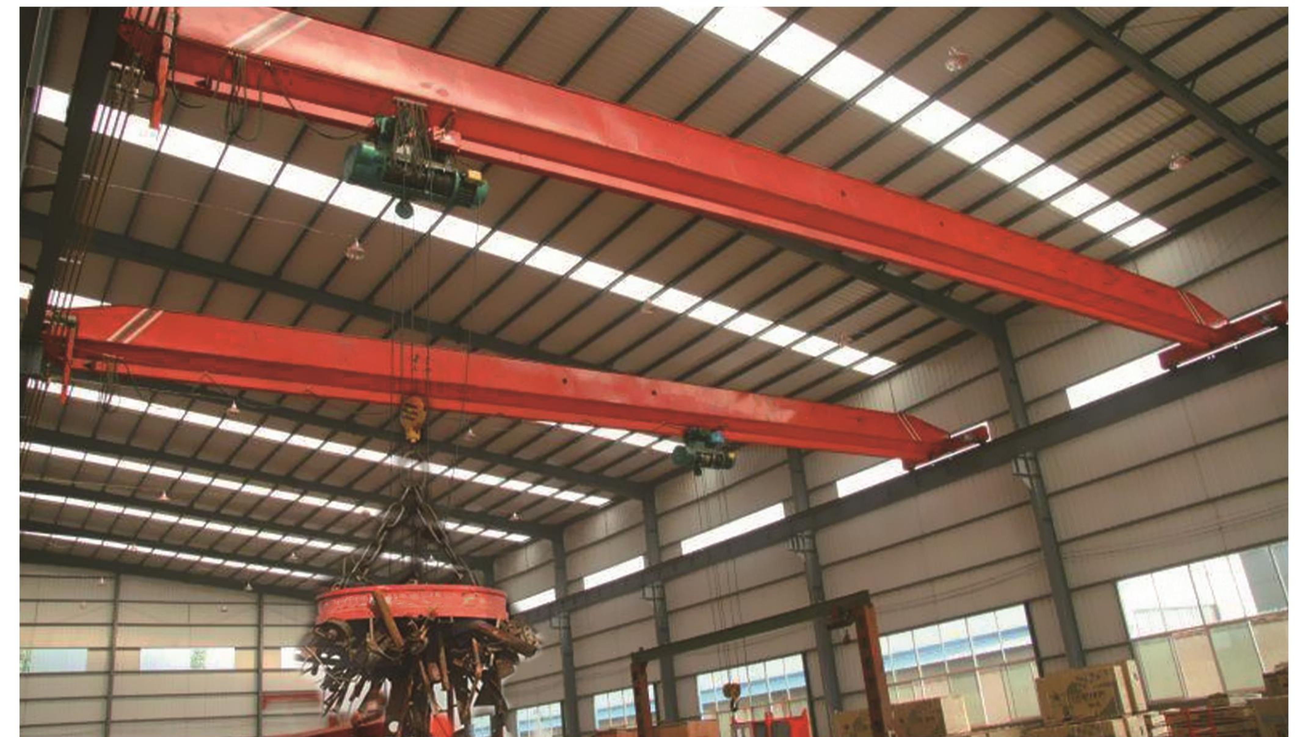
Single beam lifting electromagnet overhead crane
